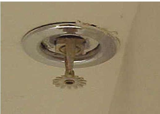
FIGURE 1. Sprinkler head installed too close to the wall.
